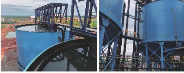
(a) Top view of the paste thickener (b) Upward view of feeding pipes
